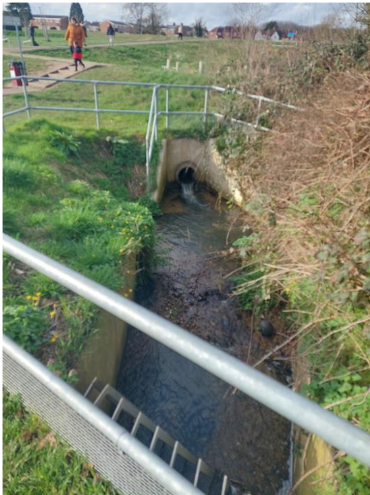
Photograph 6: View of stream passing through Harts Hill Playground and entering culvert on opposite side of Chapel Street
