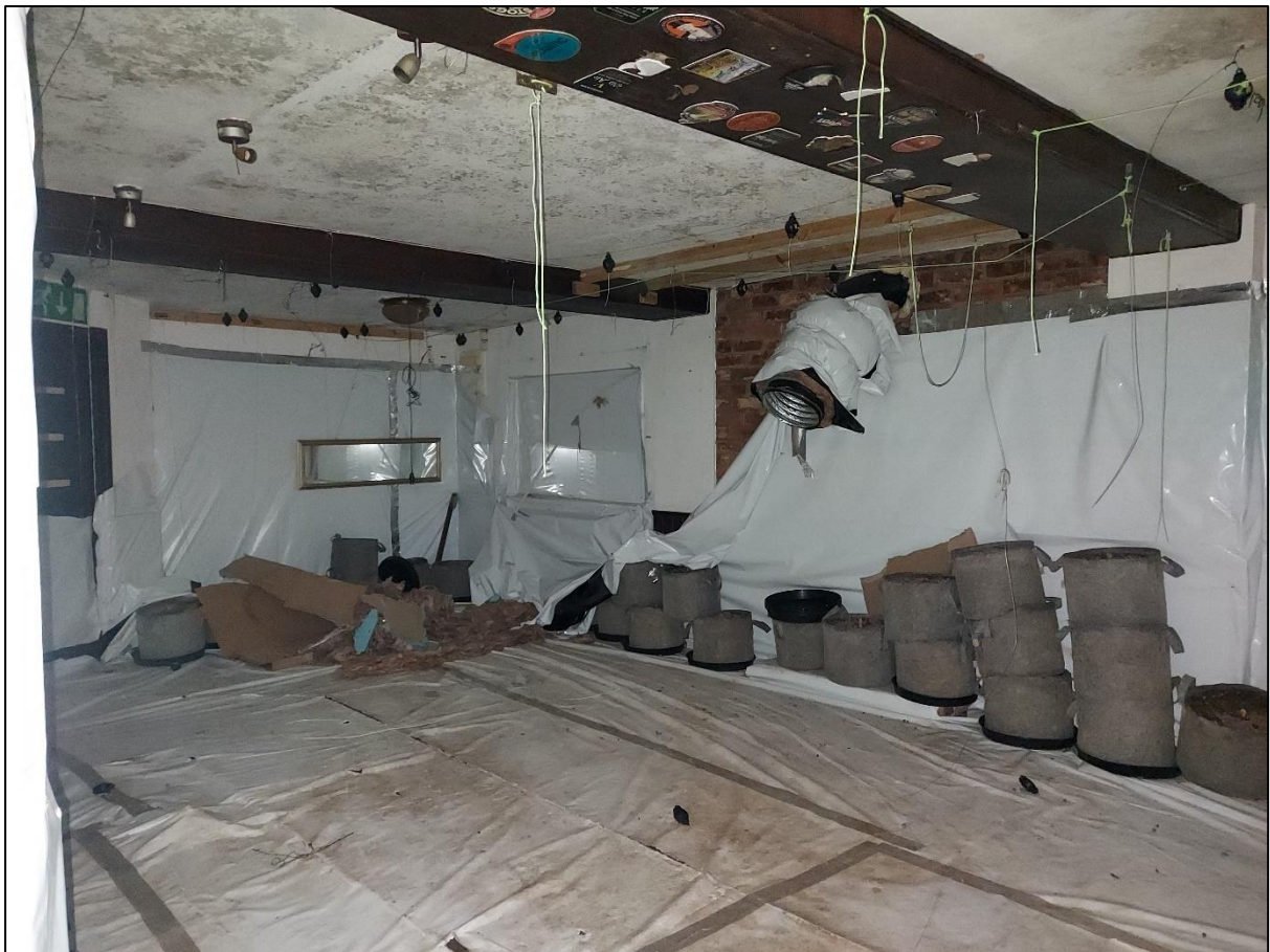
Photo 6: Fireplace obscured and damaged by recent vent
